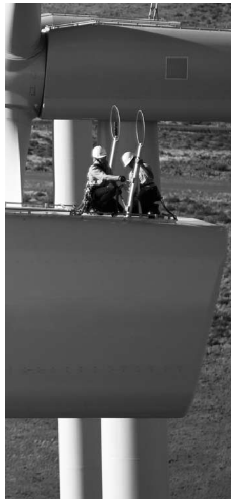
Anchorage on wind turbines often are improperly located.
